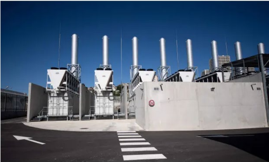
📷 A data centre in France. Such energy-intensive facilities are deemed prime candidates for heat recycling. Photograph: Clement Mahoudeau/AFP/Getty Images
